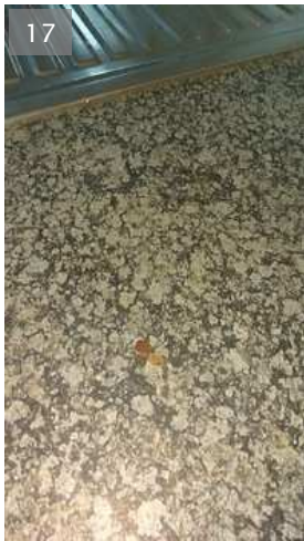
Counter top damaged - surface broken 24/02/2018 09:49 (SAST)
