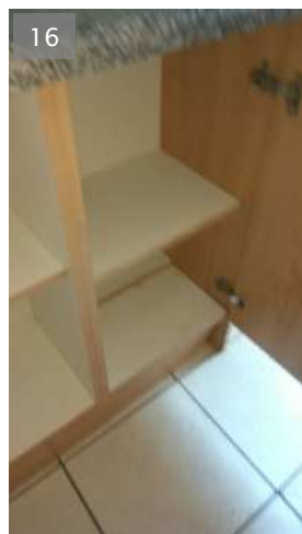
Kick board and side panel loose. 24/02/2018 09:47 (SAST)
